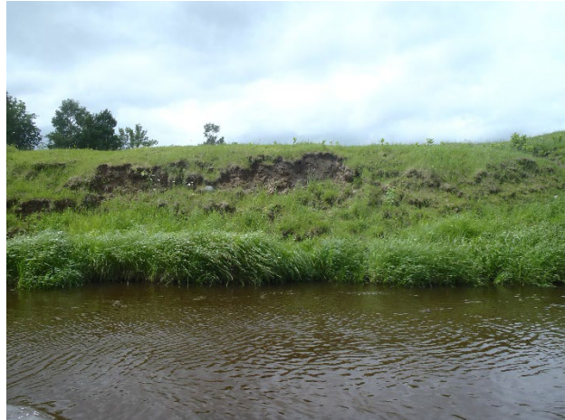
Erosion in LOW County
