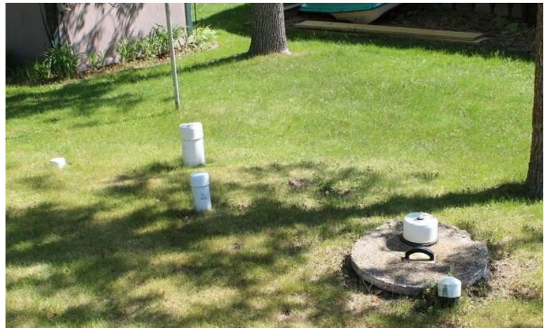
Septic system on a lake lot
