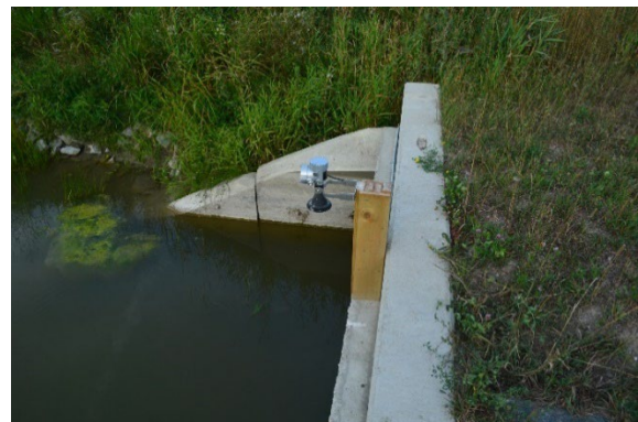
Water Level Monitor, Bostic Creek Planning Region
